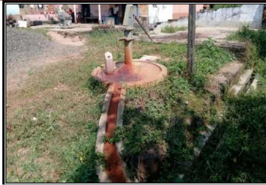
Photo Plate No: - 1 High Iron Affected Tube Well in Taldangra Block.
